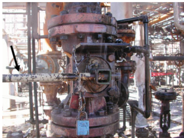
Figure 2. The shut-off valve and valve wrench (indicated by arrow on far left). [Color figure can be viewed in the online issue, which is available at www.interscience.wiley.com .]
